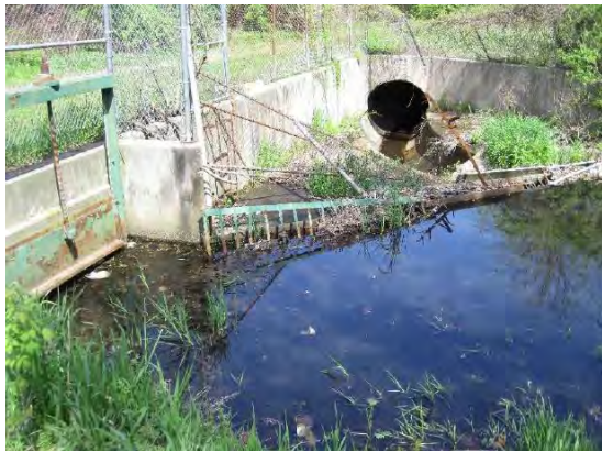
The Hockanum Diversion Structure behind Silver Lane Plaza is in need of repairs
